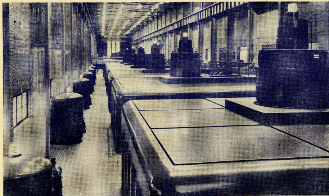
Generator Room in Shipshaw No. 2 Power Plant, 12 units, 1,200,000 hp, 208 ft. head. A stop-off to visit this development has been arranged on the Saguenay Boat Trip
