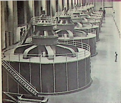
An interior view of the Nevada wing of Hoover Power Plant in the Las Vegas Section area, showing seven generating units in operation. Each generator is rated at 82,500 kilowatts, and each turbine is rated at 115,000 horsepower.
