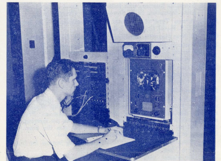
TV Test Panel, Northwestern Bell Telephone Co.
