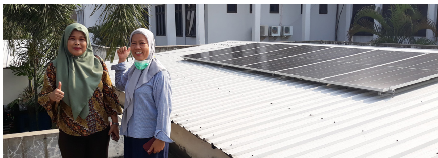
IEEE Team members delight in the completion of the on-grid roof top photovoltaic power plant in Jakarta, Indonesia.
