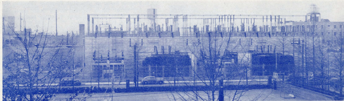
Jamaica Substation, Consolidated Edison Company, which may be seen on Monday and Tuesday afternoons
