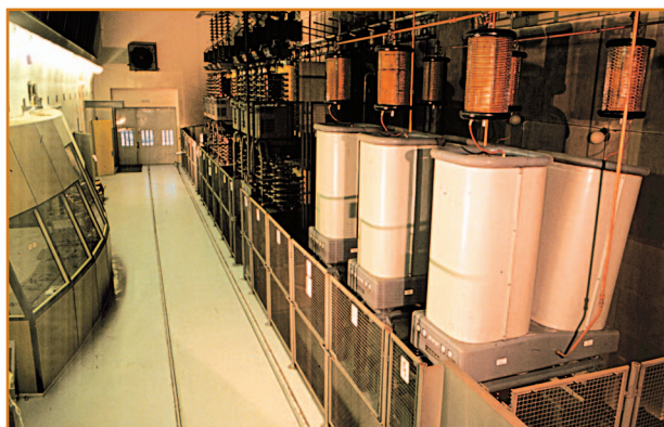
figure 5. Gotland Converter Station with mercury arc and thyristor valves.
