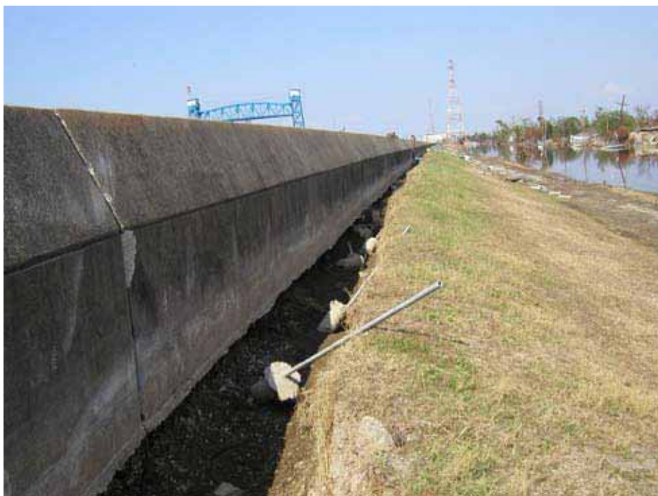
Figure 5. Scour from overtopping along the Inner Harbor Navigation Canal (Photo Credit: U.S. Army Corps of Engineers, IPET)
