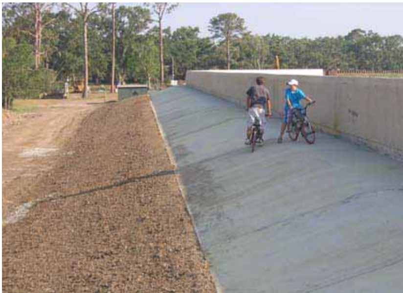
Figure 6. Floodwall with new splash pad, Orleans Avenue Canal (Photo Credit: John McQuaid)
