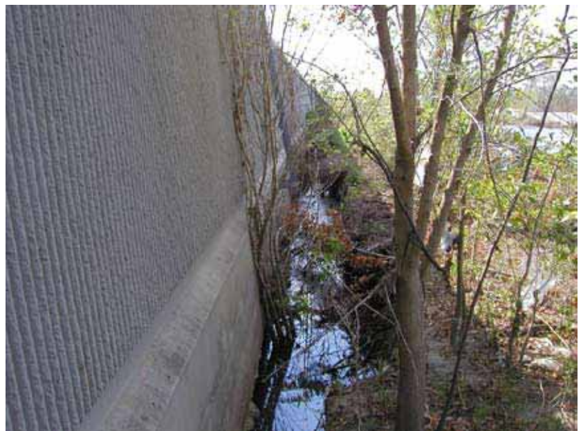
Figure 4. Water -filled gap along London Avenue Canal (Photo Credit: U.S. Army Corps of Engineers, IPET)
