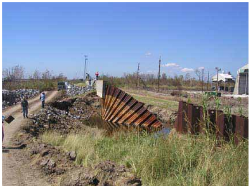
Figure 7. Transition failure along the New Orleans East back levee (Photo Credit: US Army Corps of Engineers, IPET)
