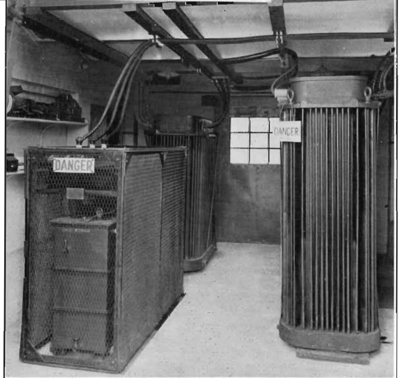
DUBILIER 100 kVA CONDENSER BANK connected to sub-station transformers
