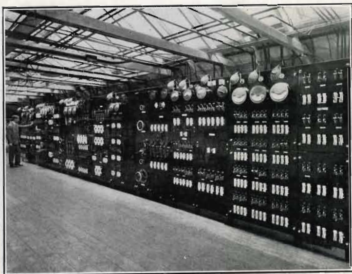
SWITCH ROOM Supplying power and light throughout the whole factory.
